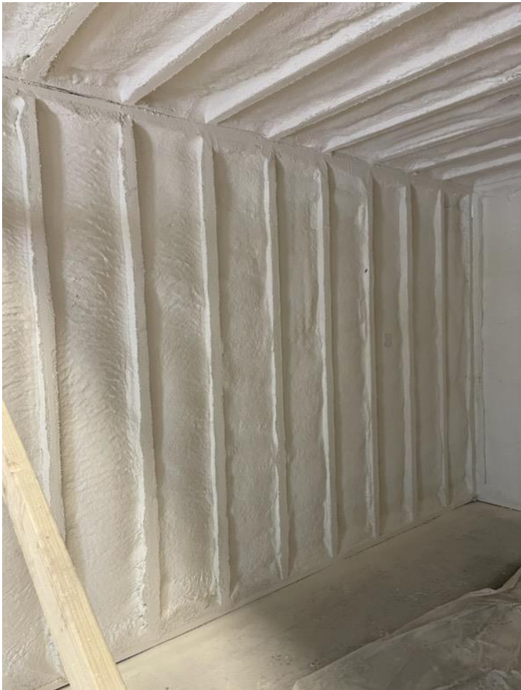
Above: Elmendorf, TX Corner Test Room coated with spray foam insulation and SafeCoat ® TBI (Thermal Barrier Innovation).
